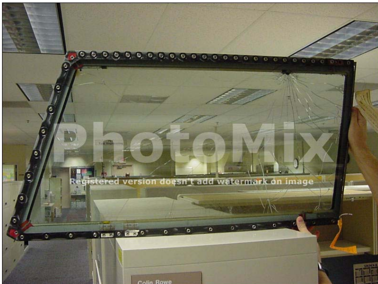
Fig 2. No 1 outer ply fractures
